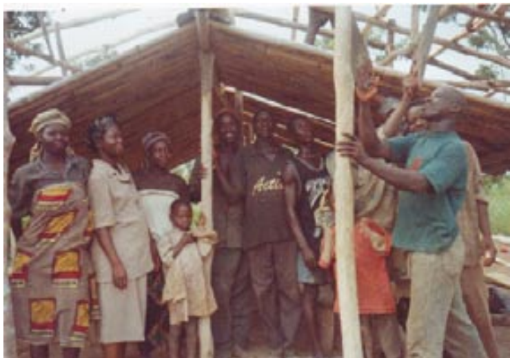
Nathaniel’s family and some of the saints building a new meeting place in a tribal village. Nathaniel is one of the early trainees, now one of the leaders and a missionary to a tribal area in the North.
